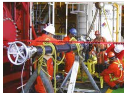
▼ CHT2000 hot tapping offshore application.
