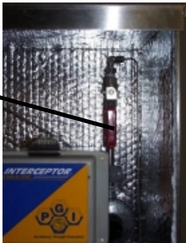
Main Gas Supply Valve "ON"
