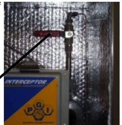
Main Gas Supply Valve "OFF"
