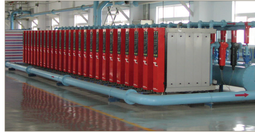
Example of a multi-bank installation
